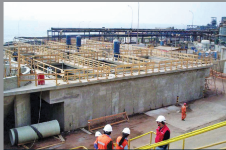
Reverse Osmosis Desalination Plant, Chile
