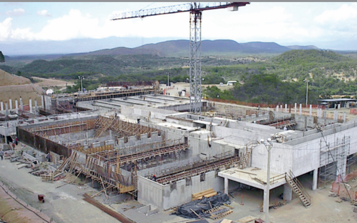
Mao Point Wastewater Treatment Plant, Dominican Republic
