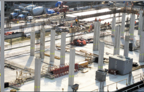
Croton UV Water Treatment Plant, USA
